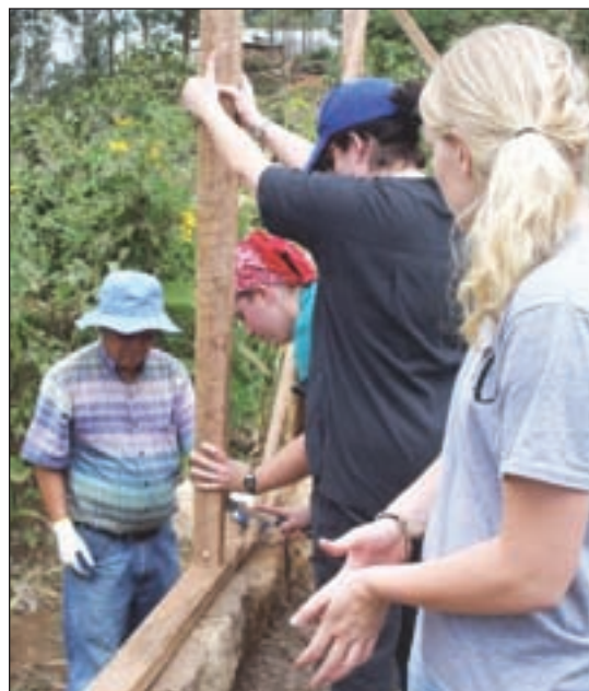
Elizabeth Reed, Karol Clay and Brittani Hays raise the walls for the AIDS orphan home in Maua, Kenya.
